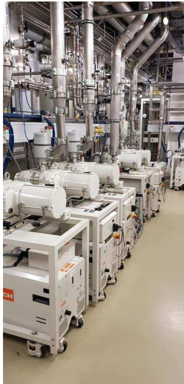
图 16. Vacuum Pumps in a Wafer Fabrication Facility
